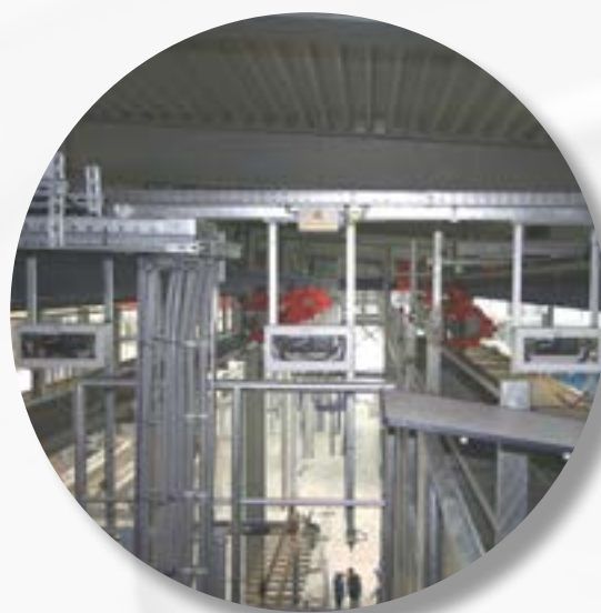
2. DATAEAGLE is located directly in the ceiling construction and is the base station (Master).
